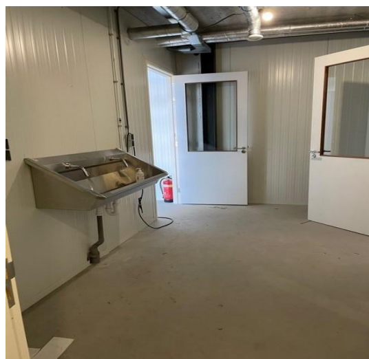
wasbakken in sanitairruimte
